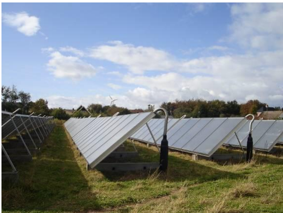
Img 4. District heating plant with solar field, Nordby, Samsø.
