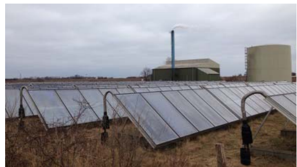
Figure 2: Nordy-Mårup district heating plant
