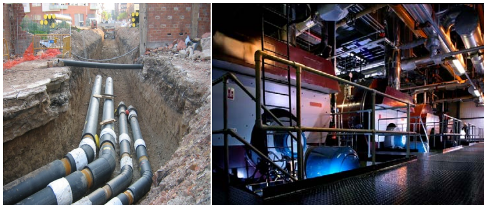
Left: District heat and chilled water mains being installed (sized to meet future requirements) and right the Energy Centre on ground floor of the car park building
