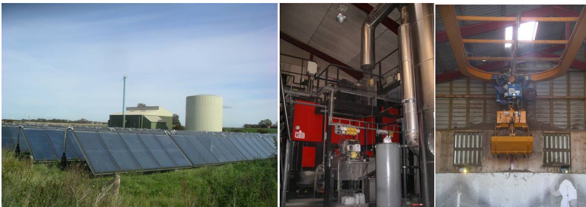
Nordby and Marup District Heating Left: Solar Farm, Boiler House and Buffer Vessel, Centre: Woodchip Boiler, Right: Automated movement of woodchip to feed hopper.
