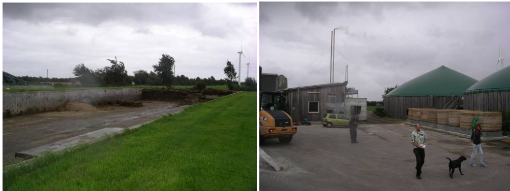
Nissen Biogas plant Left: one of a number of feed stores, Right: First and second fermentation vessels and controls house
