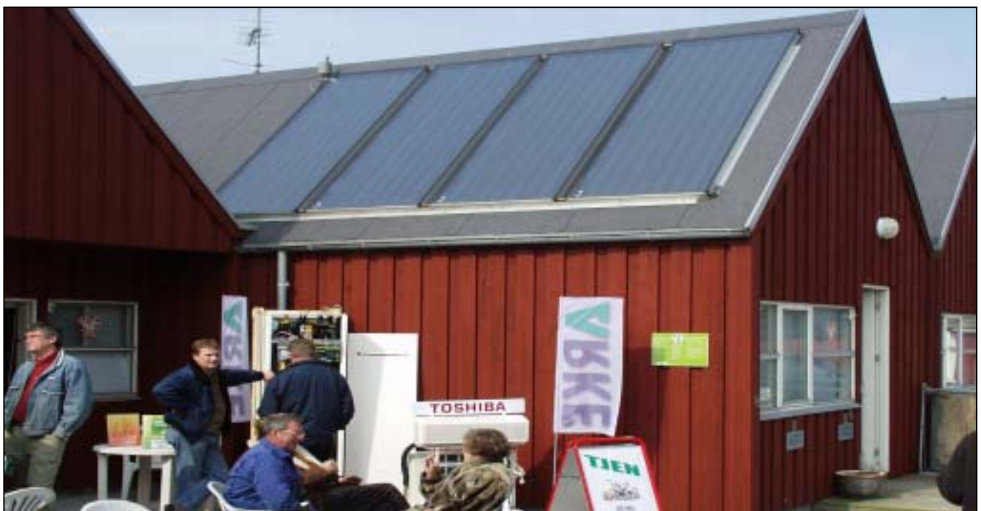
Solar heating system in Mårup Harbour
