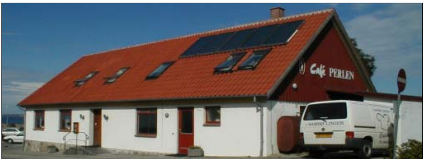
Solar heating system at Café Perlen in Sælvig
