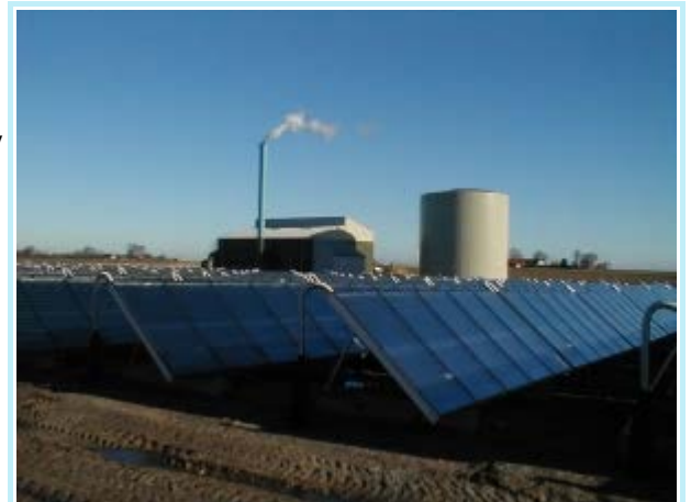
The Nordby-Maarup plant. Solar array in the foreground. Accumulation tank (round) and boiler house (with chimney) in the background.
