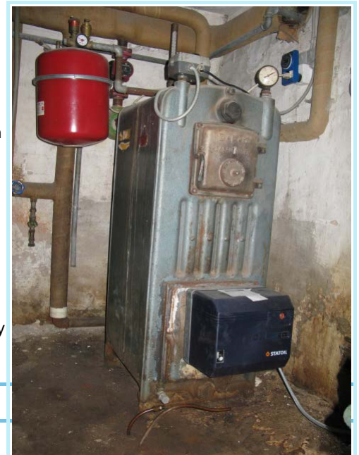
Fig. 1 Oil boiler. The black box at the bottom is the furnace (Statoil), and the tall blue container is the boiler (DFJ Salamander C). The furnace is new, but the boiler is old and not insulated, with low efficiency.
